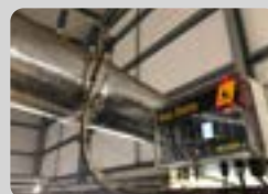
Gas Flow Monitoring
